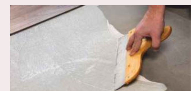
Cracking at corner & around cuts may be caused by improper conditioning, improper bonding, poor planning, avoid all these to prevent cracking at corners.
